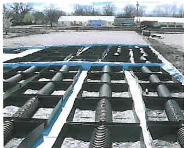
The patented subirrigation system ECS is placed at a depth of 30 cm. Slitted pipes that achieve irrigation and drainage through the same pipe system are positioned centrally inside PVC trays that measure 1.5 m x 1.5 m and are surrounded by 13 cm high sidewalls.
